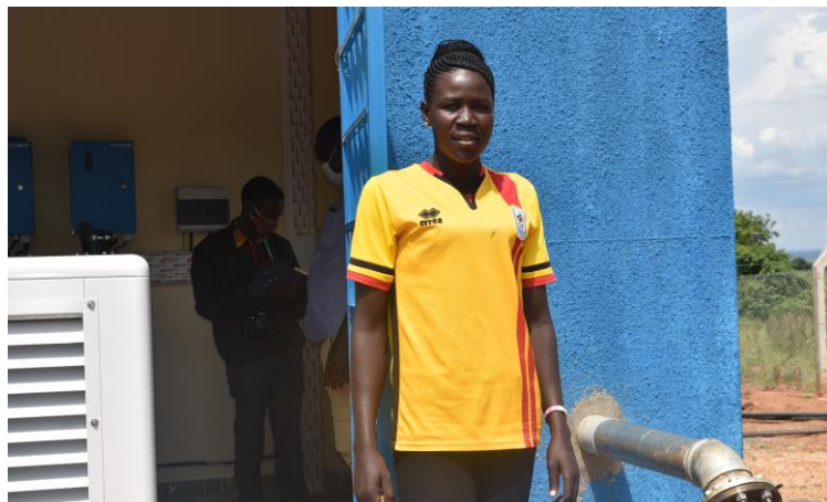
Halima at Pawor water supply station in Madi Okollo District.
